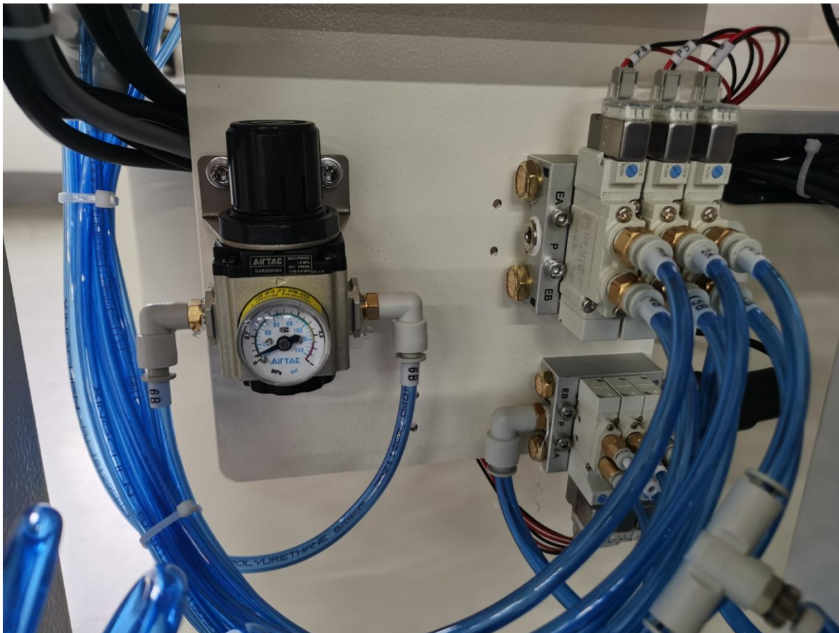
The valve is used to control the feeding group, with a factory setting of 0.05MPa
